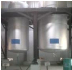
Steam Condensing Unit
