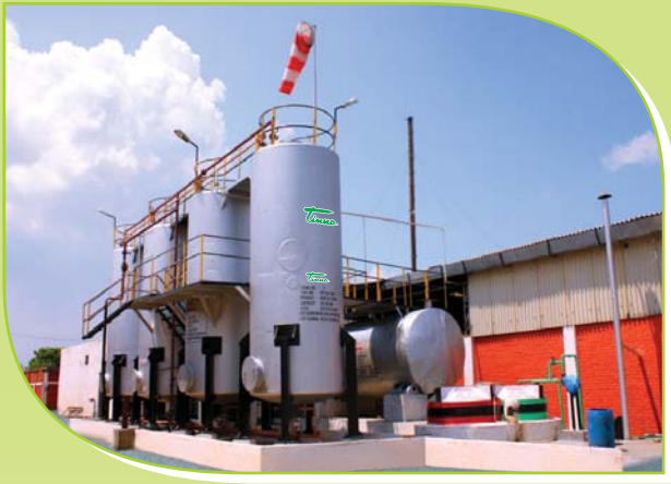
Bitumenous Products Plant
